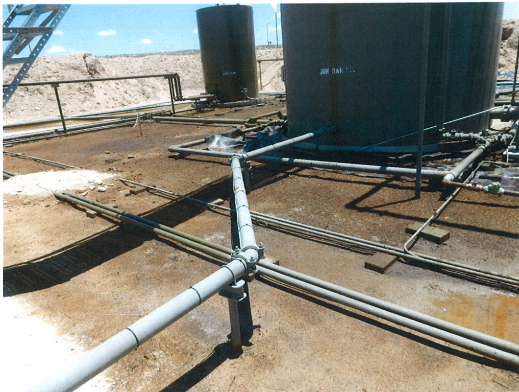
New Spill (June 14, 2017) Viewing Southeast, June 27, 2017
