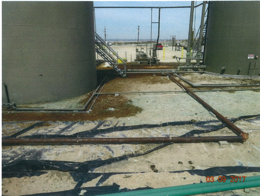
Spill Area Viewing North
