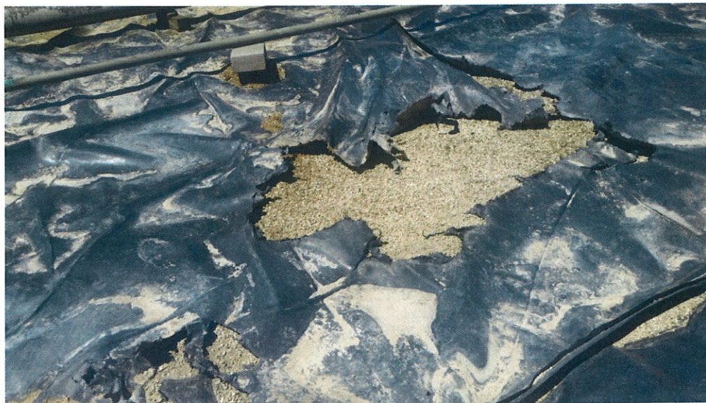
Break in Liner South of Tanks May 12, 2017
