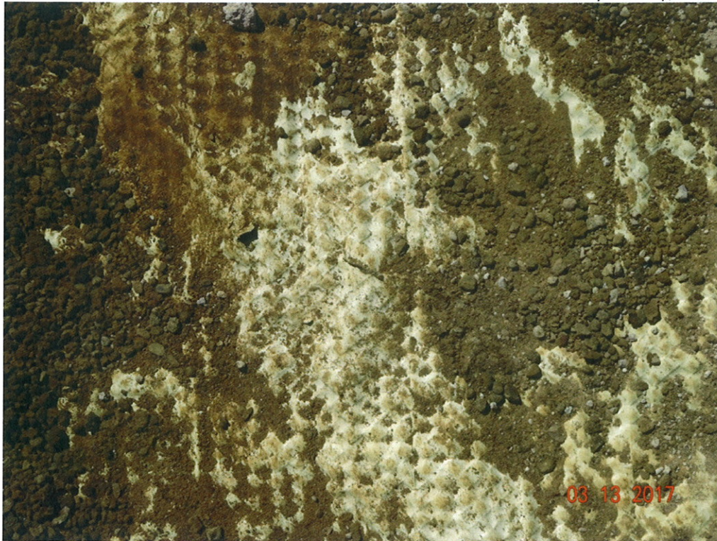
Small Tear in Bottom Liner inside Firewall
