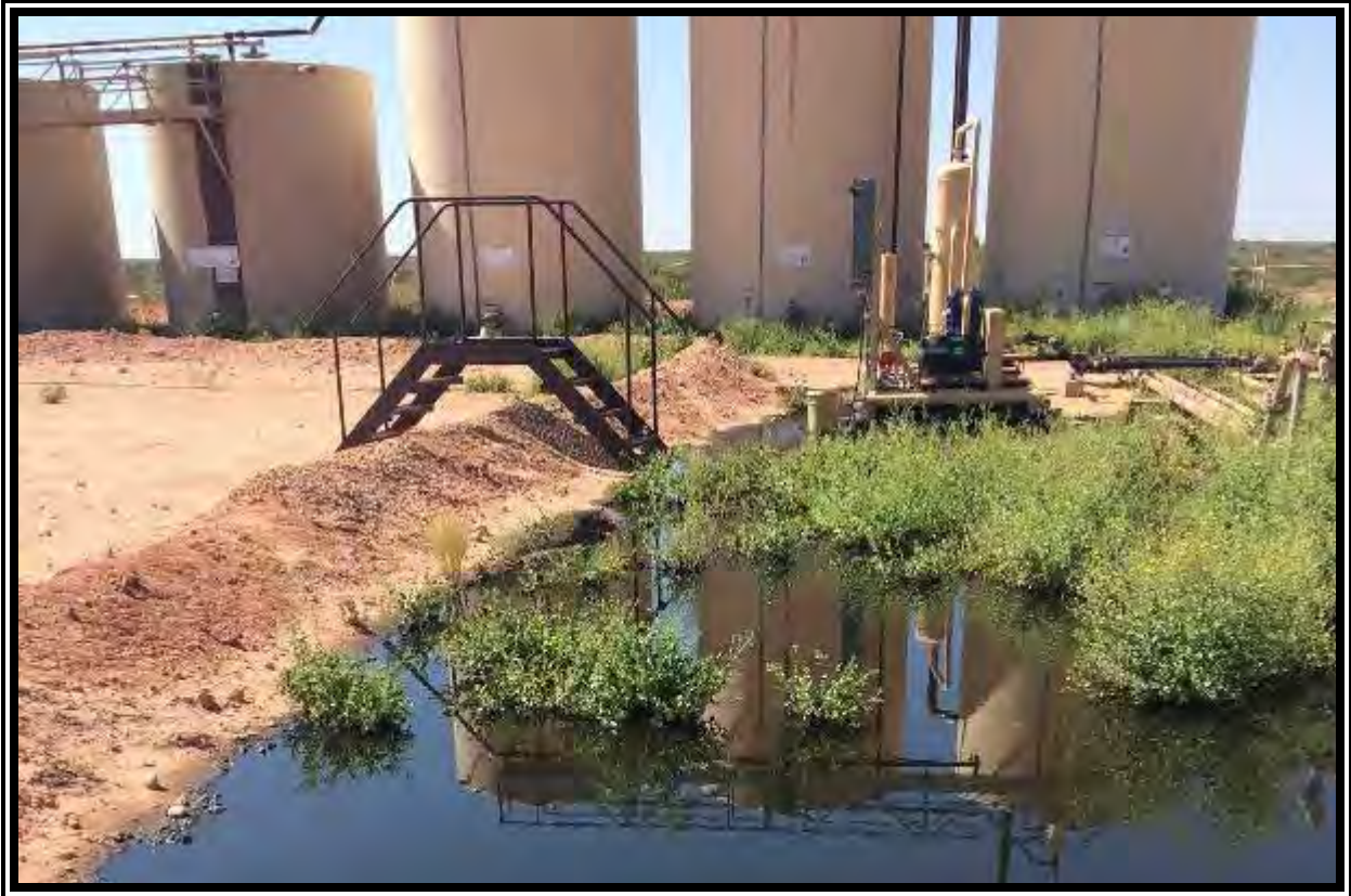
View of pooled oil north of tank battery containment.
