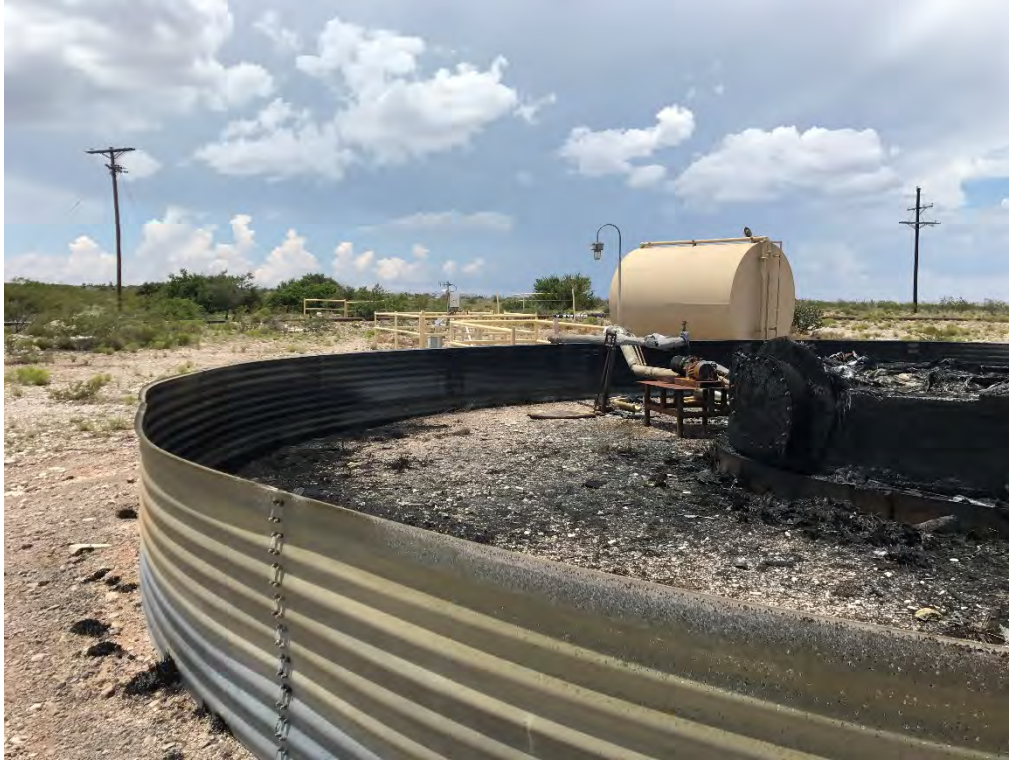
Indian Basin Station 210 – Release (Looking Northwest)
