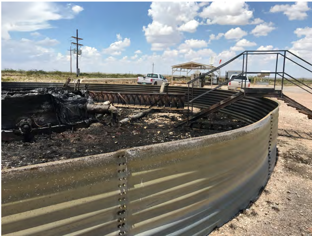
Indian Basin Station 210 – Release (Looking North)
