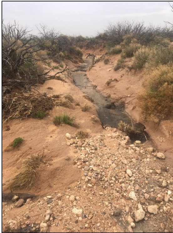
PHOTO 5: View of release in draining / creek bed, facing north west. 3/21/2019
