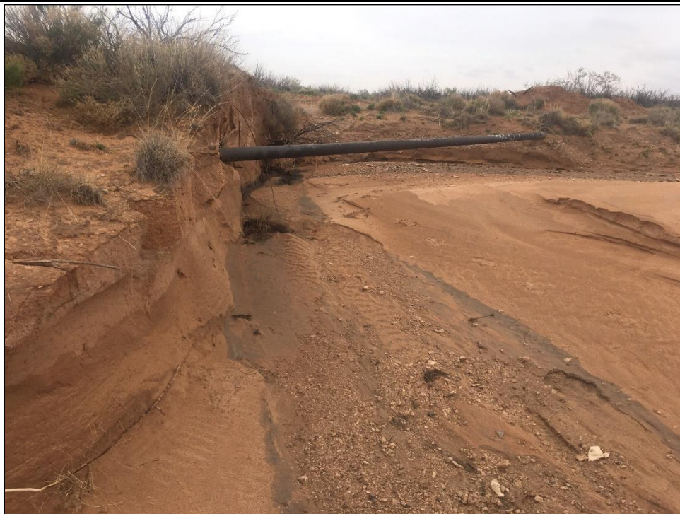
PHOTO 6: View of release in draining / creek bed bend, facing north. 3/21/2019
