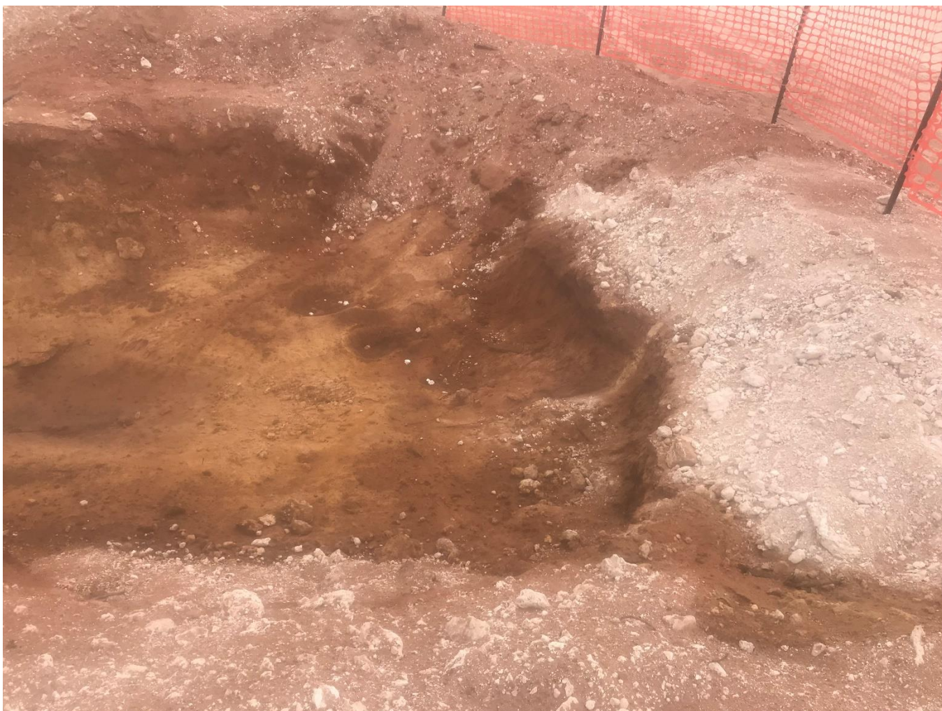
Soil surrounding the point of release during site assessment activities.
