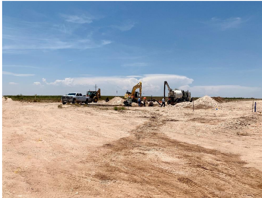
Photo 1: Initial Release Surficial Path – looking NW at Release Point
