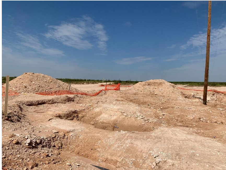
Photo 10: Area Around Electrical Pole and Burnt Surface – looking NW at pole
