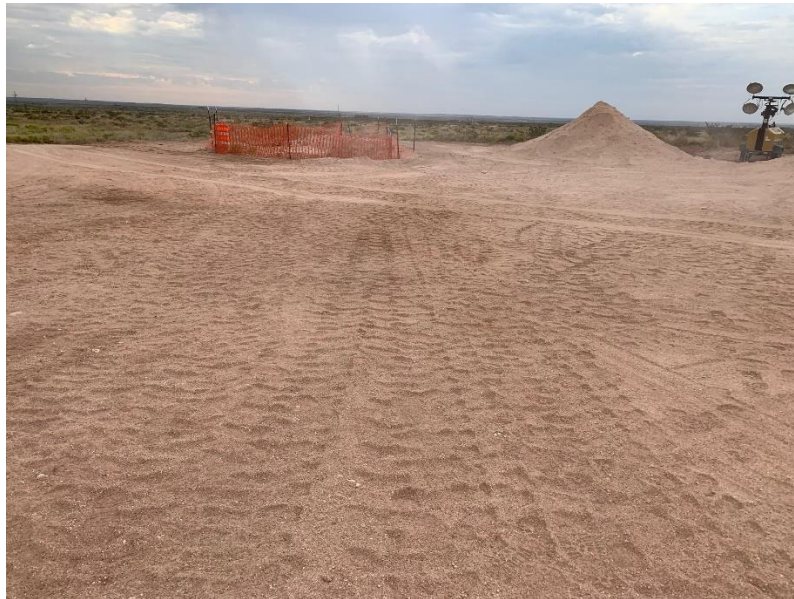
Photo 19: Restoration of Access and Area Around Electrical Pole– looking SE at final excavation area and clean caliche backfill pile
