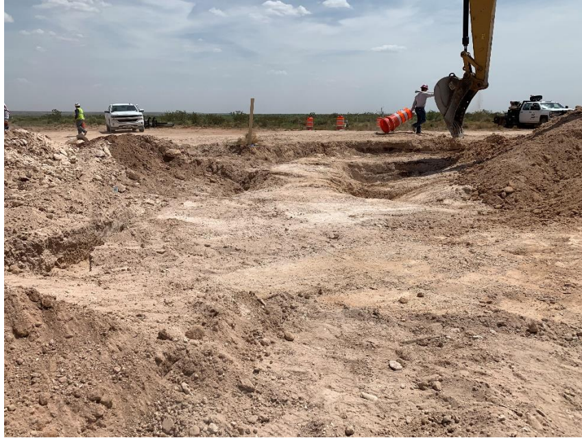
Photo 9: Area Around Electrical Pole and Burnt Surface – looking South
