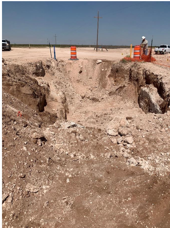
Photo 14: Off Right of Way Excavation – looking NW toward release point (electrical pole in distance)
