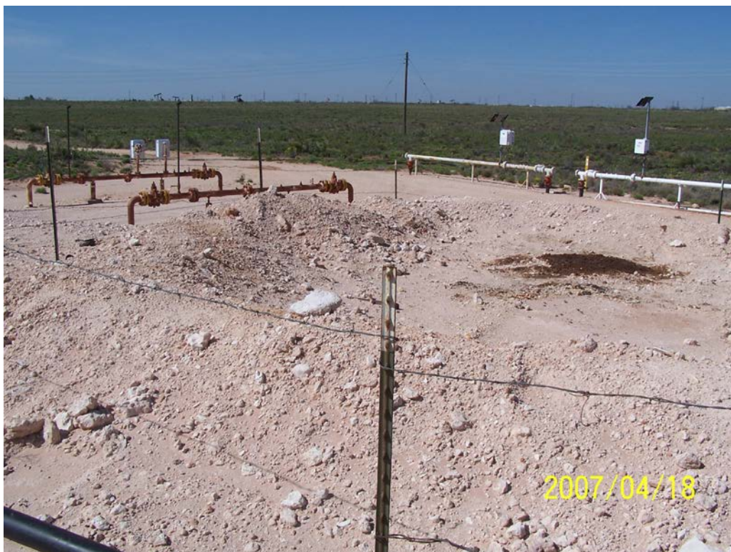
Photograph No. 4 – Looking south at tank battery bermed area (south end) and meter runs.
