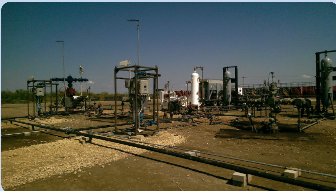
Compact MPFM Installation, South Texas
