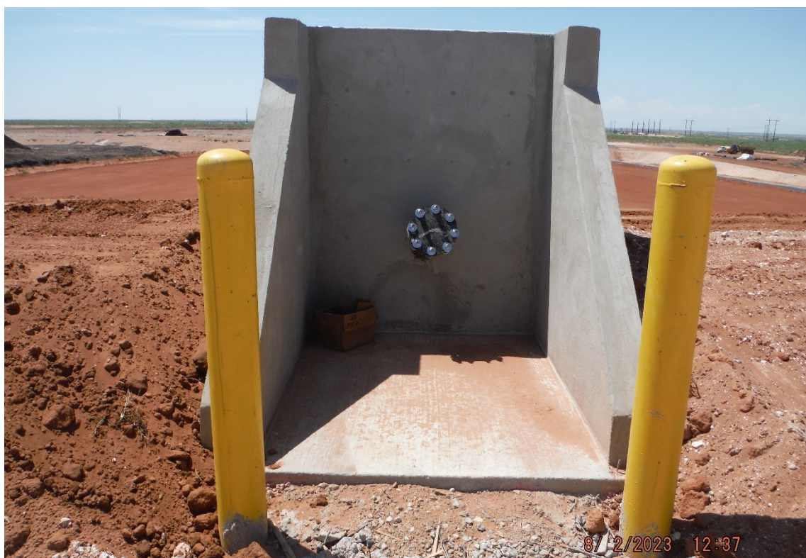
2023-08-02: Leachate Access Structure
