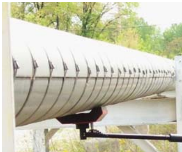
Figure 2 Detection of Moisture in Insulation using Neutron Backscatter
