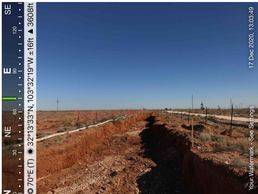
View East, of impacted area
