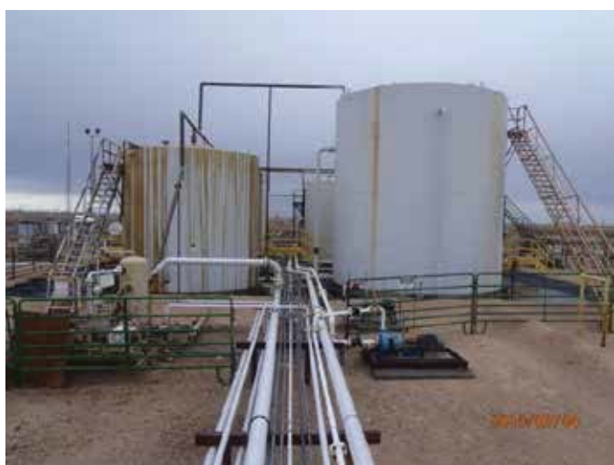
Initial release area, facing north 3/4/15
