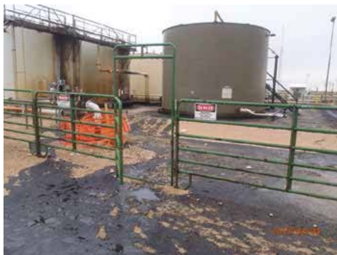
Initial release area, facing north 3/4/15
