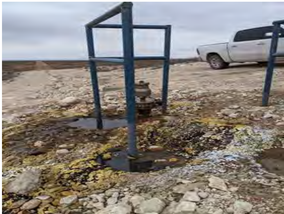
Photo 1: View of pipeline release source at air relief valve (ARV) facing west down right-of way
