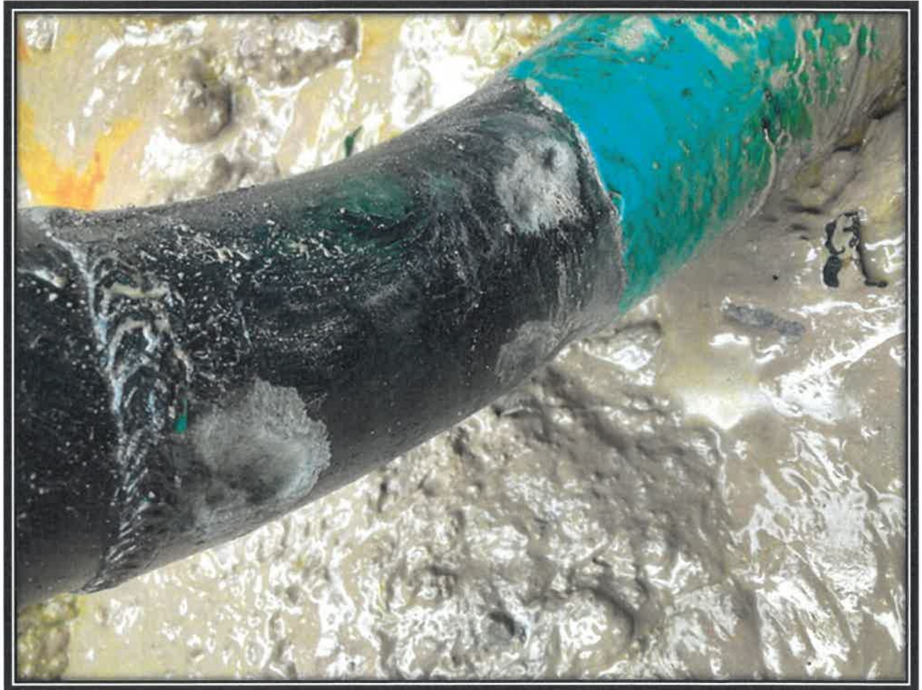
Photo 2: Failure of Flowline
