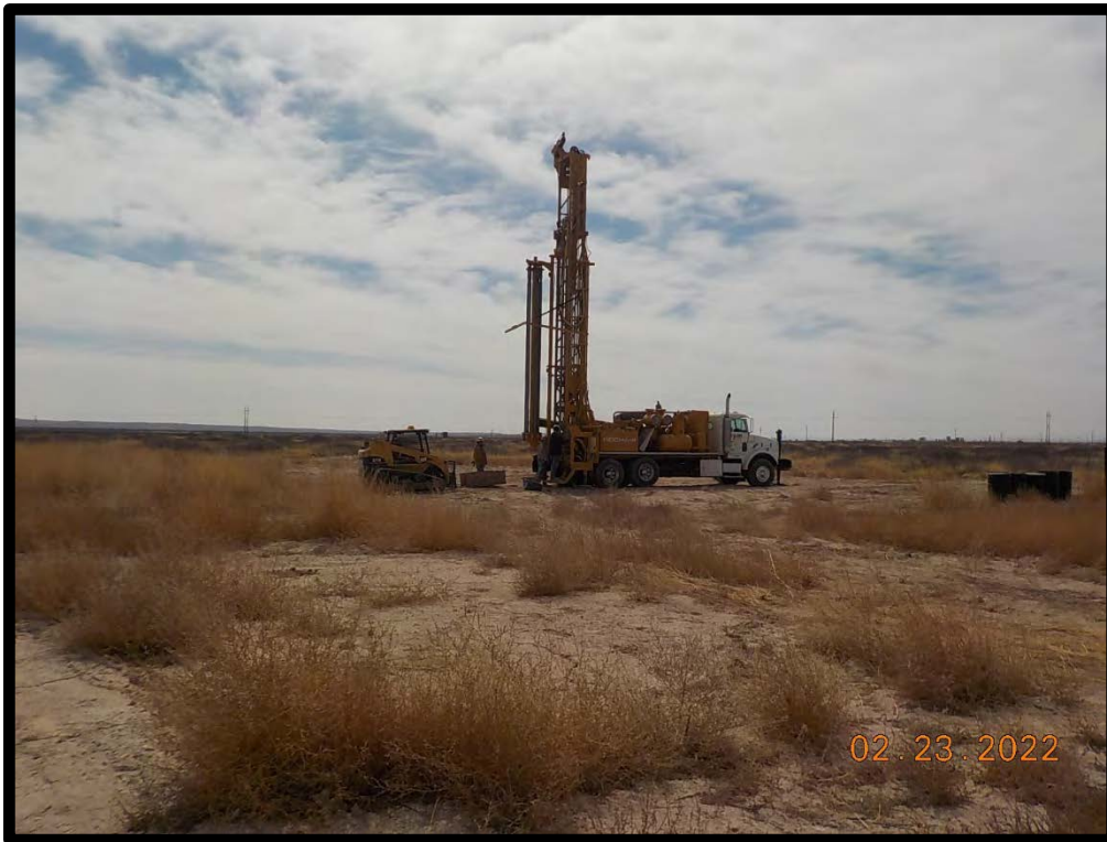
PHOTOGRAPH NO. 3 – A view of the air rotary soil boring installation activities at the “SB-1” location on February 23, 2022. The view is towards the southwest . (Approximate GPS: 32.724414, -104.346120)
