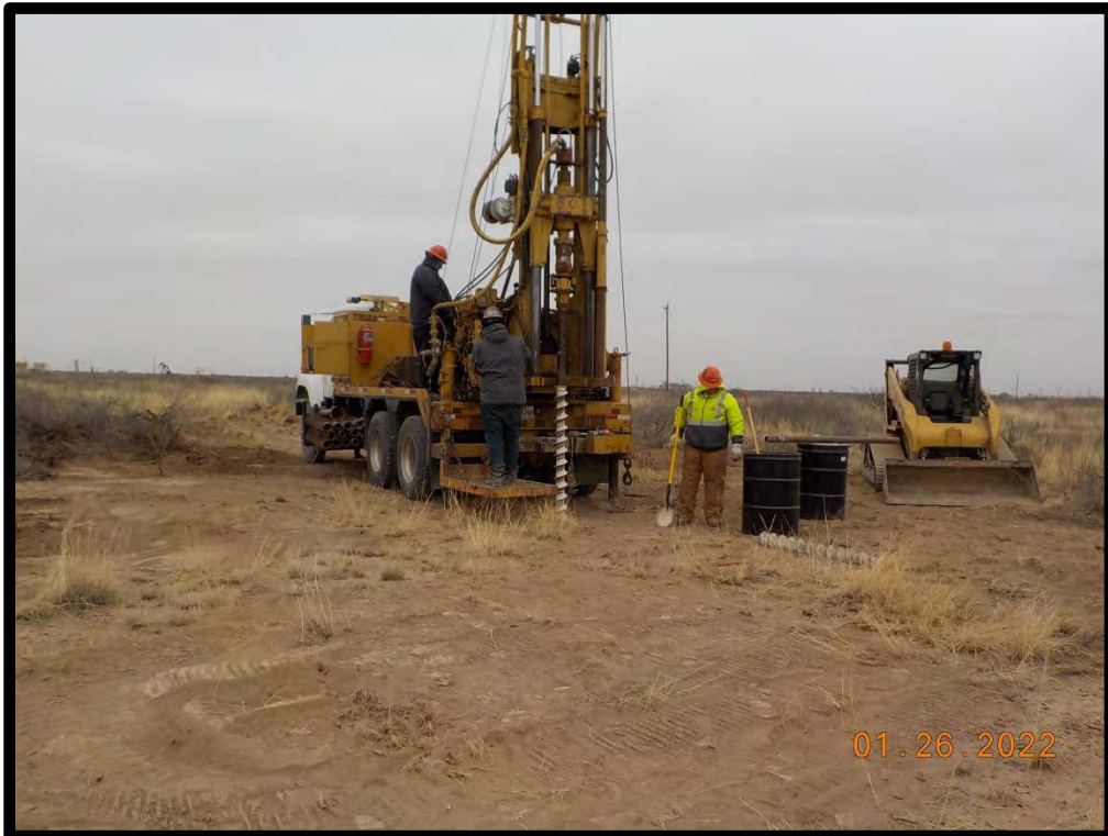
PHOTOGRAPH NO. 2 – A view of the attempted background soil boring on January 26, 2022. The view is towards the northeast.
