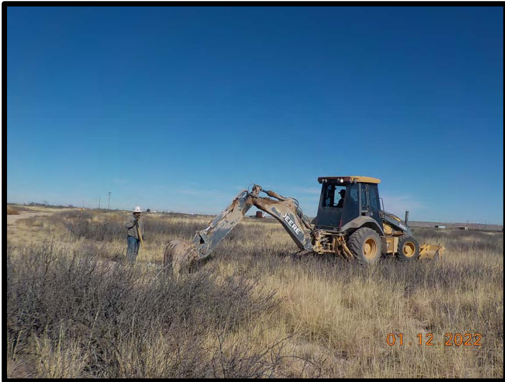
PHOTOGRAPH NO. 1 – A view of the horizontal assessment activities in the vicinity of test excavation “NNE-2.A” on January 12, 2022. The view is towards the north-northeast.
