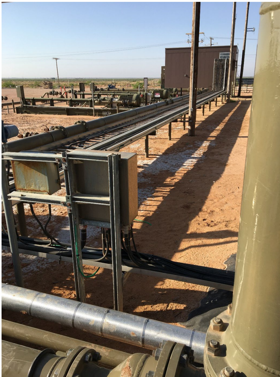
Impacted area viewing southeast, May 20, 2021
