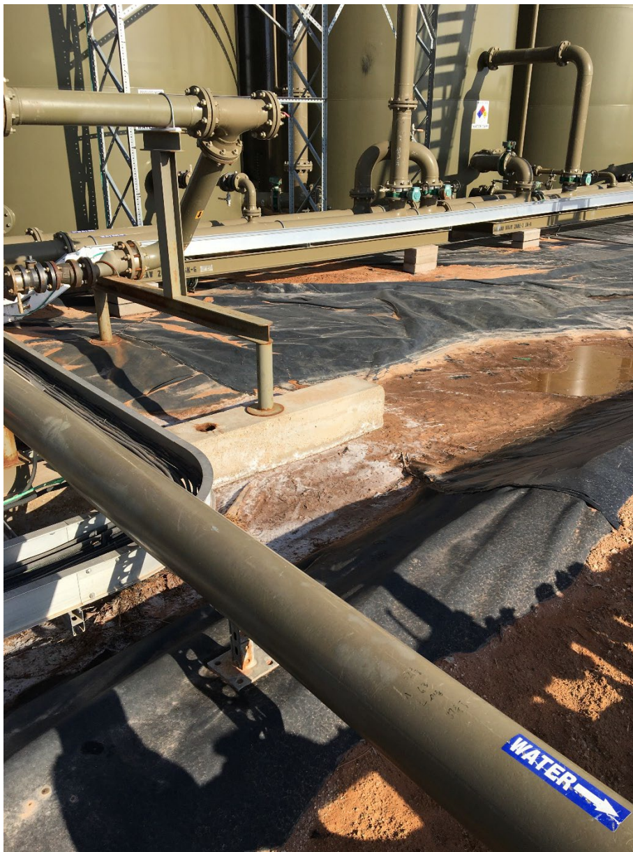
Impacted area viewing northwest, May 20, 2021
