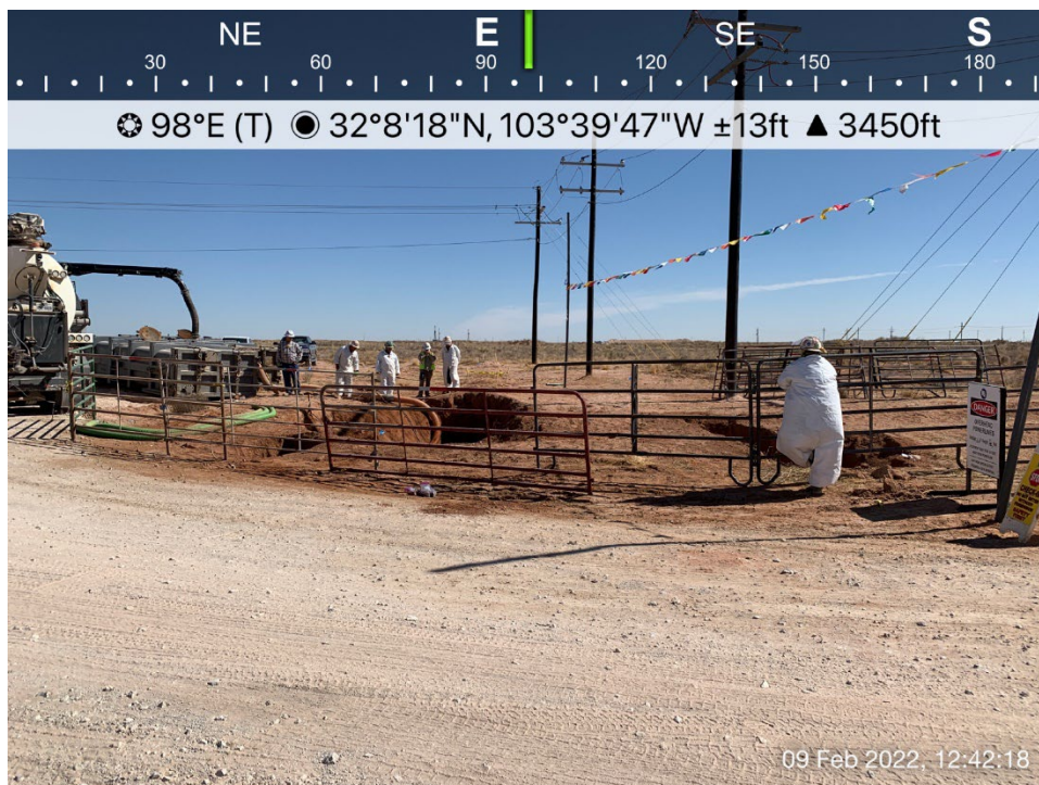
Impacted area viewing east, February 9, 2022
