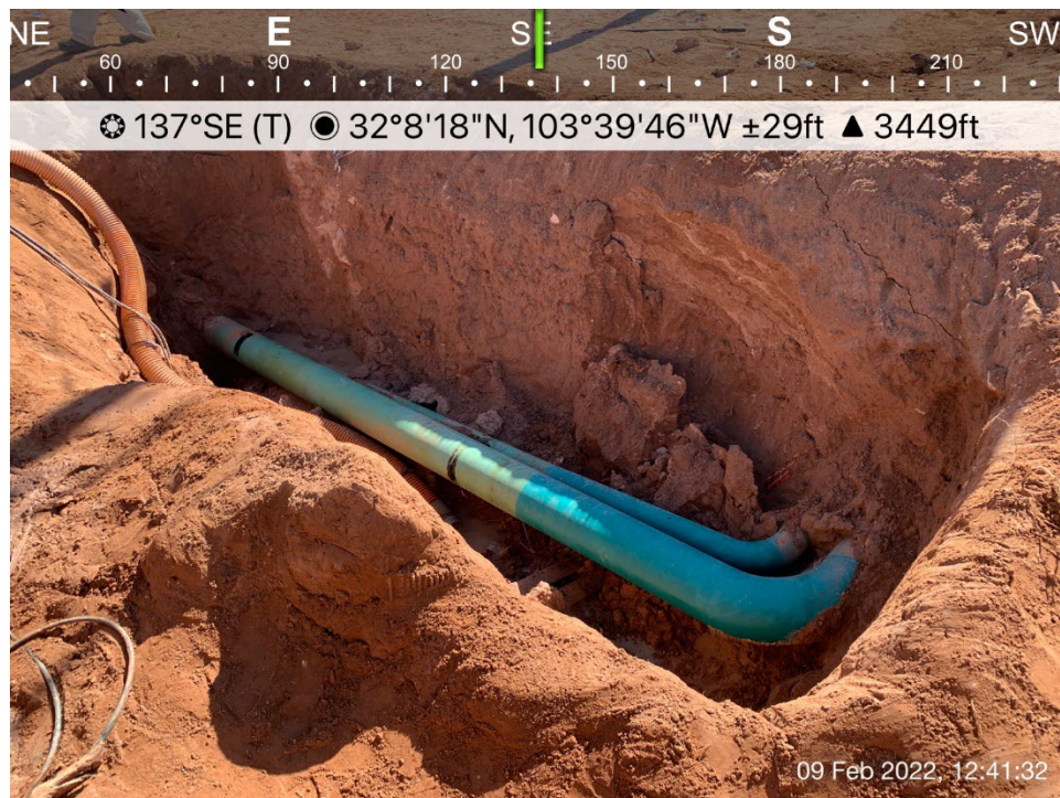
View of impacted line, February 9, 2022
