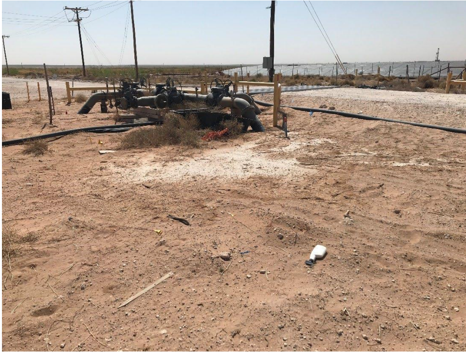
Impacted area (nAPP2211732512) viewing southeast, April 18, 2022
