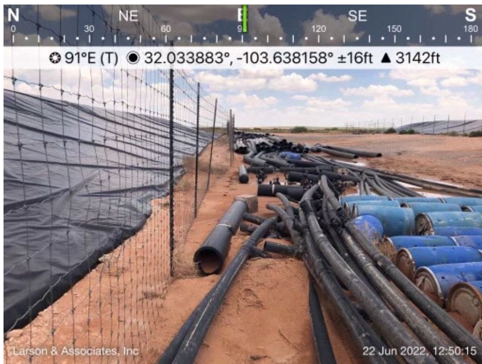
Impacted area viewing East, June 22, 2022
