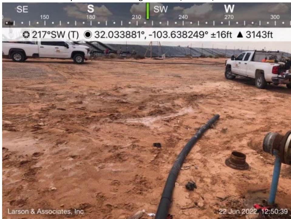
Impacted area viewing southwest, June 22, 2022
