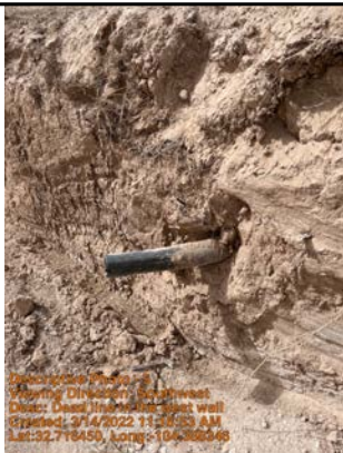
Dead line in the west wall
