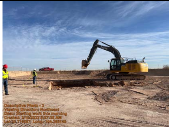
Viewing Direction: Northeast
