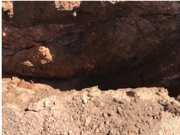
Photograph 7: View of the sidewall of pothole.
