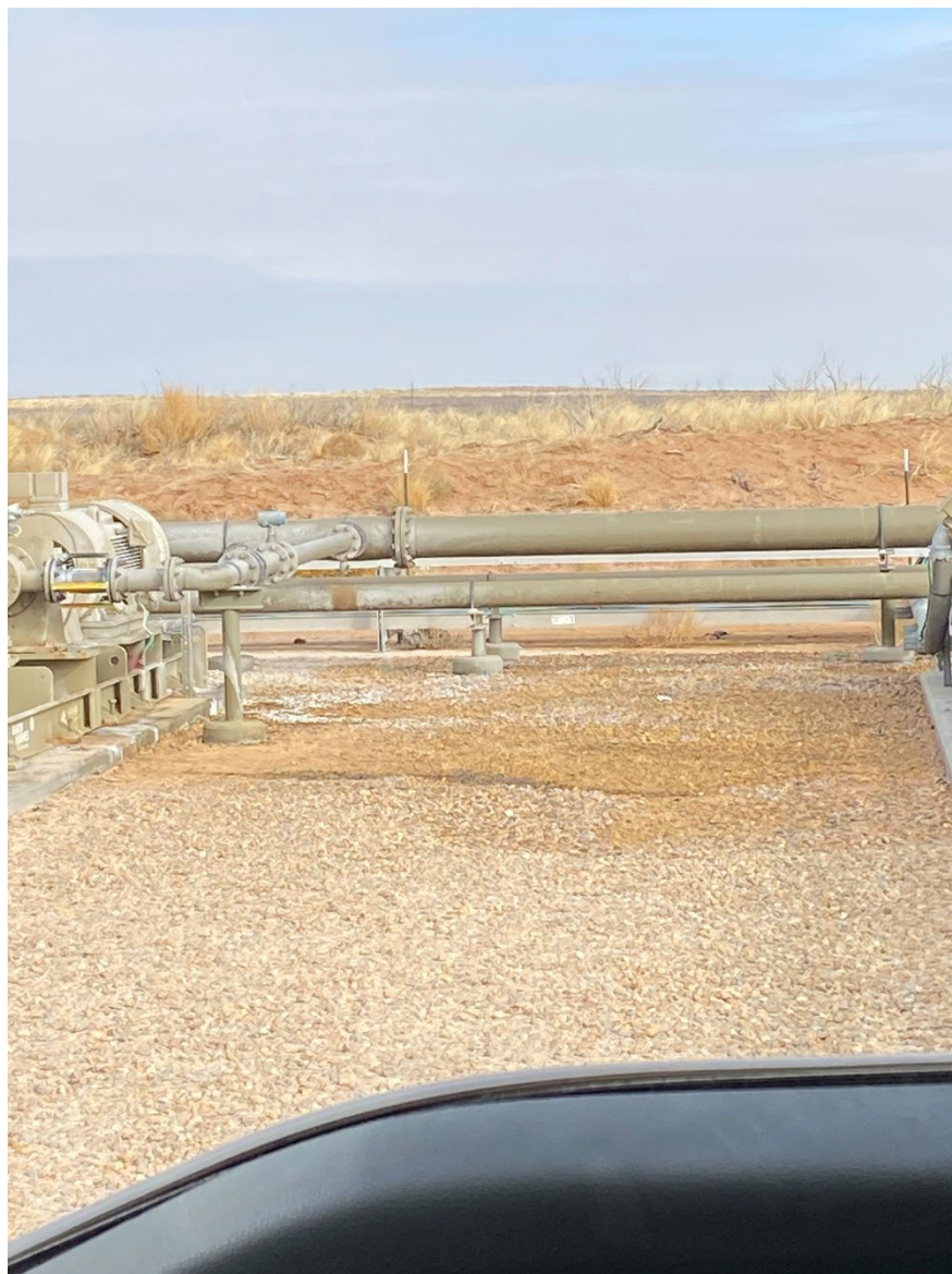
Impacted area (nAPP2202549943) captured by Chevron personnel
