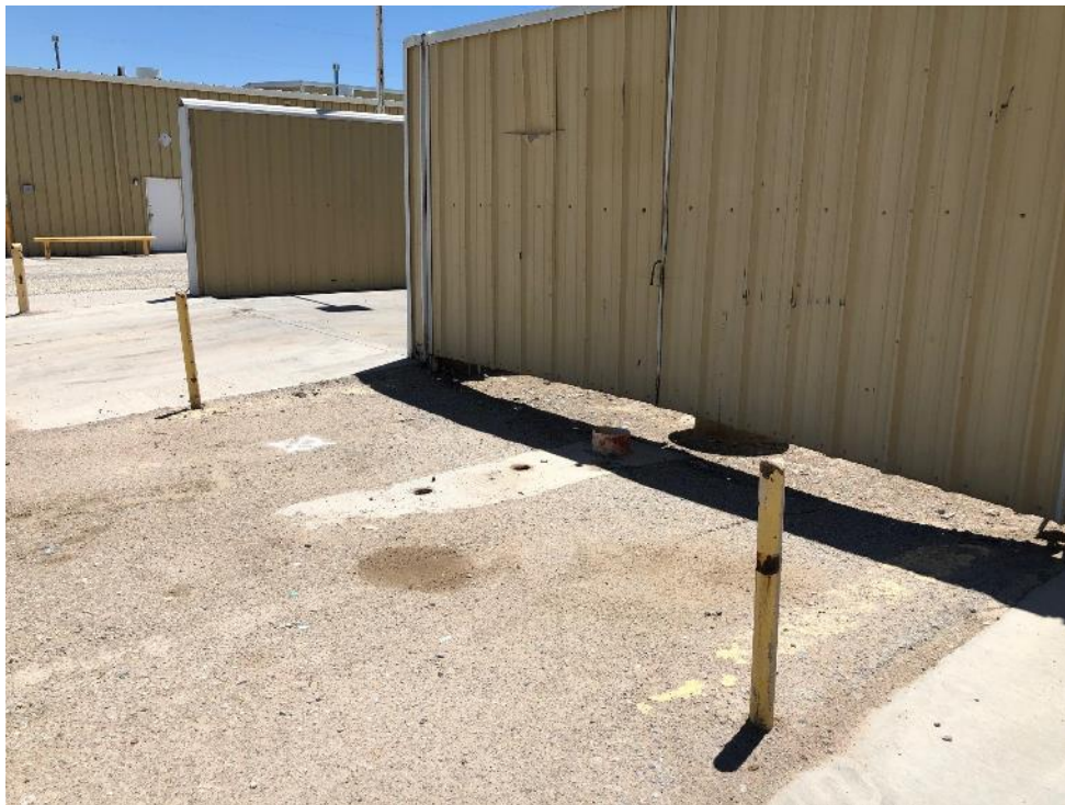
Photo 7 - Looking southeast at north end of oil water separators/grit pit at DP-12 location marked in white
