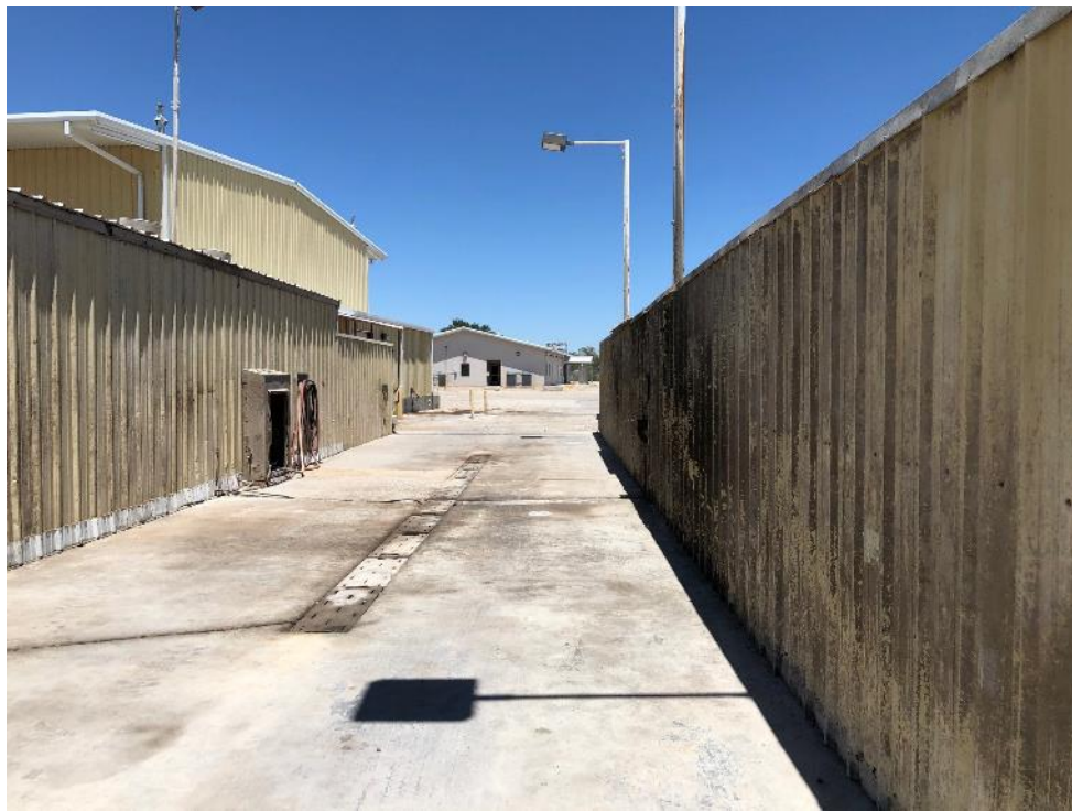
Photo 5 - Looking north through west wash bay at location of DP-8 in front of DP-9 marked in white
