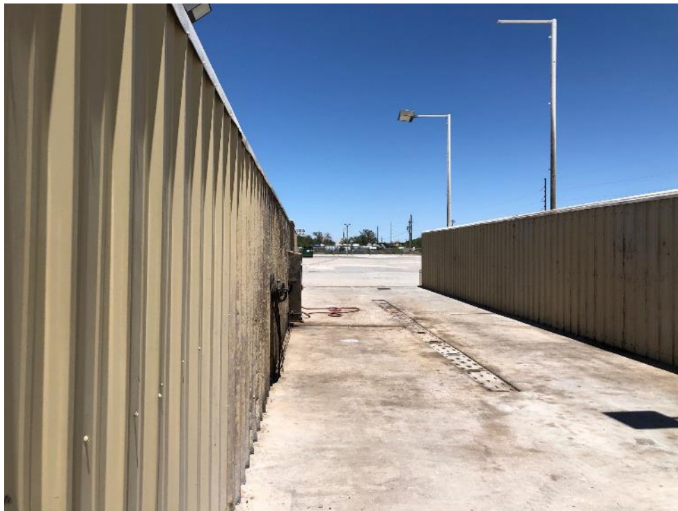
Photo 8 - Looking north through east wash bay at locations marked in white DP-14 in front of DP-13 just beyond the hose
