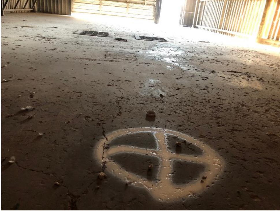
Photo 15 - Looking west at location of DP-22R marked in white inside of Building 6
