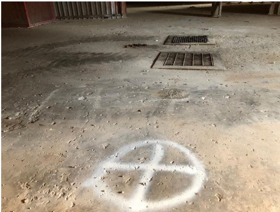
Photo 13 - Looking south at location of DP-20R marked in white inside of Building 6
