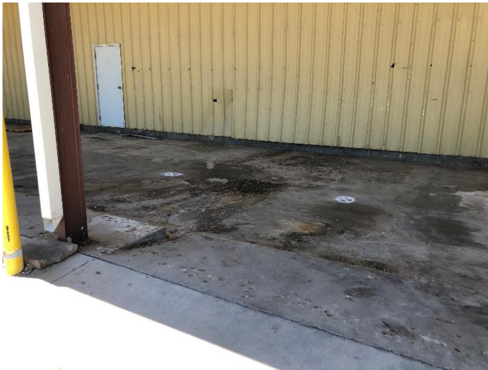
Photo 3 - Looking southwest at east side of Building 4 at DP-5 on the right and DP-6 on the left marked in white
