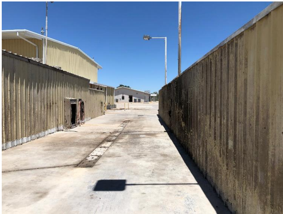
Photo 5 - Looking north through west wash bay at location of DP-8 in front of DP-9 marked in white
