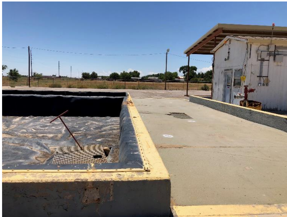
Photo 2 - Looking south at locations of DP-3 nearest containment and DP-4 near drain in truck bay. Final location of DP-4 was offset to the east.
