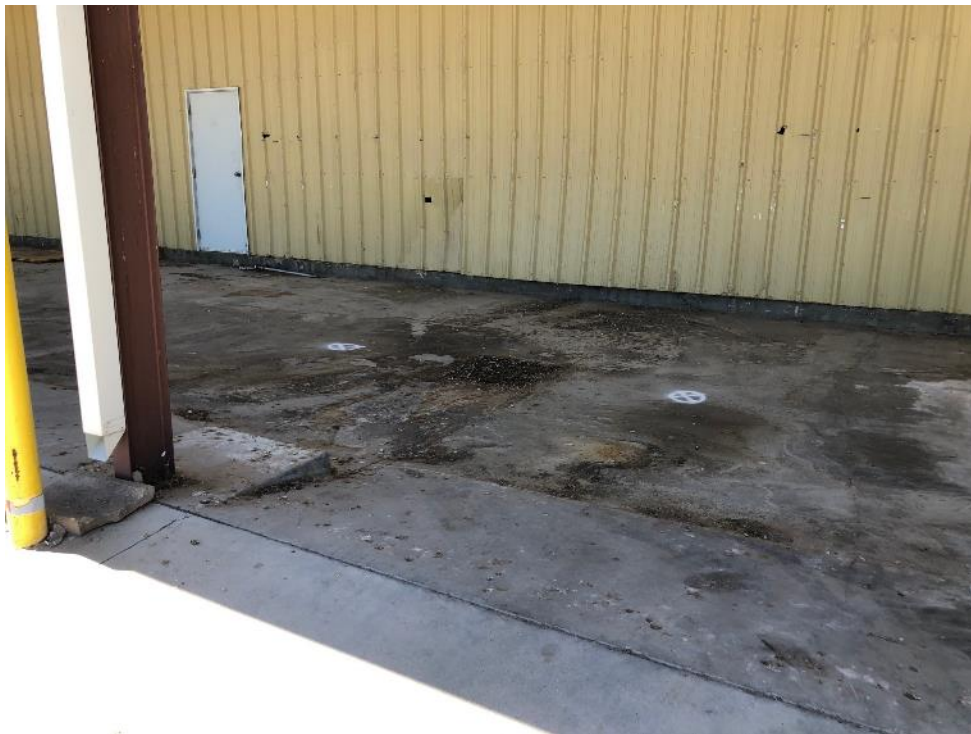
Photo 3 - Looking southwest at east side of Building 4 at DP-5 on the right and DP-6 on the left marked in white
