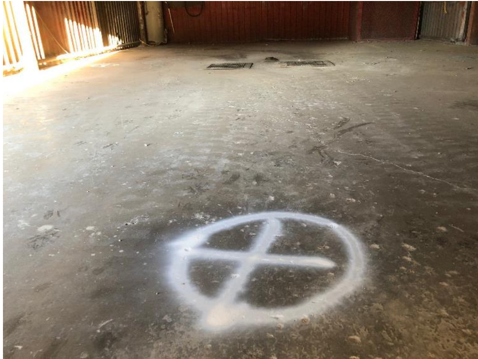
Photo 17 - Looking east at location of DP-24R marked in white inside of Building 6
