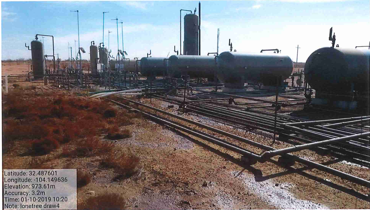
North side of spill area
