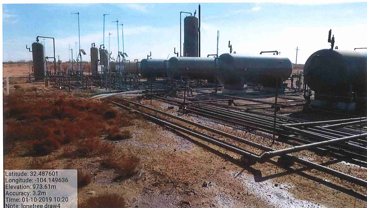
North side of spill area
