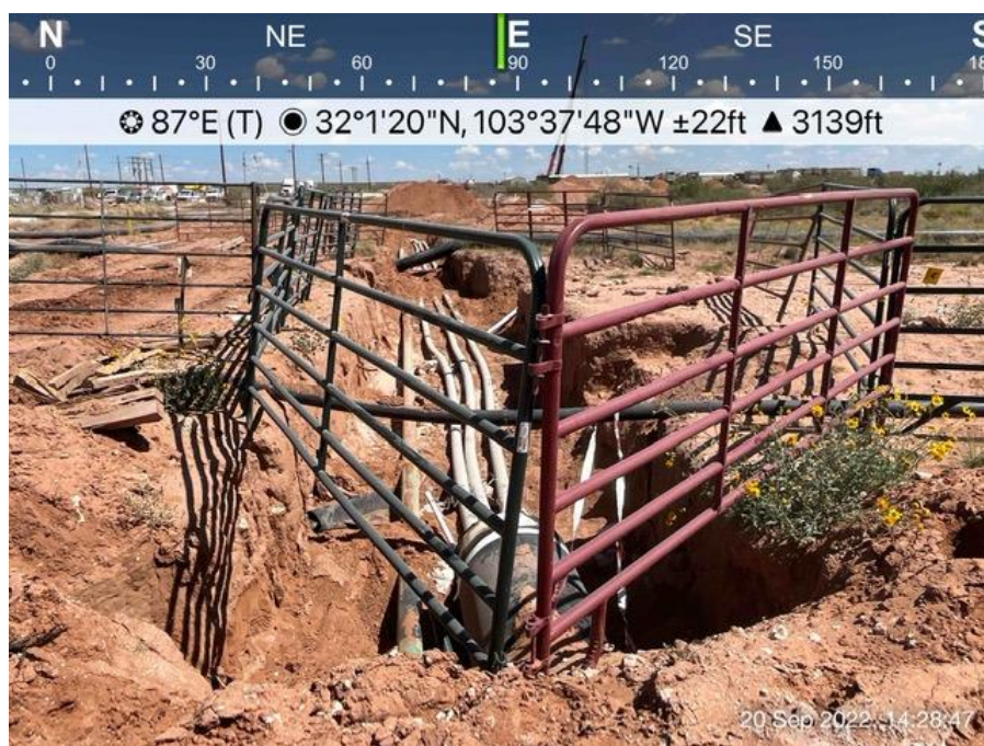
Impacted Area view showing exposed pipes from the east September, 20, 2022.
