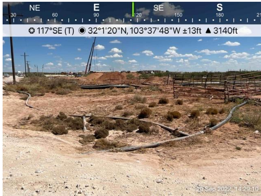
Impacted Area view showing exposed pipes from the east - southeast September, 20, 2022.
