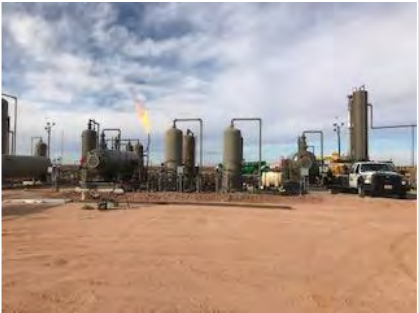
View west of bermed process equipment area
