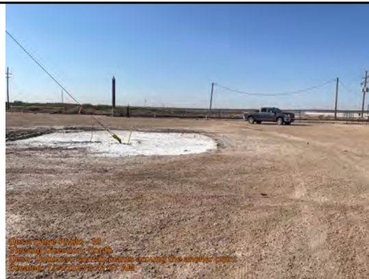
Unknown contaminants around the anchor point
