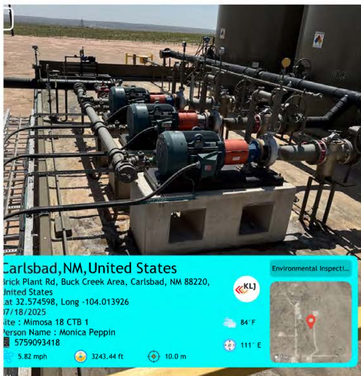
North end of containment facing west near transfer pumps.
