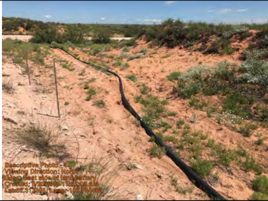
East side of tank battery
