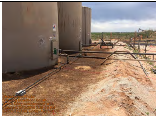
Dirty containment area
