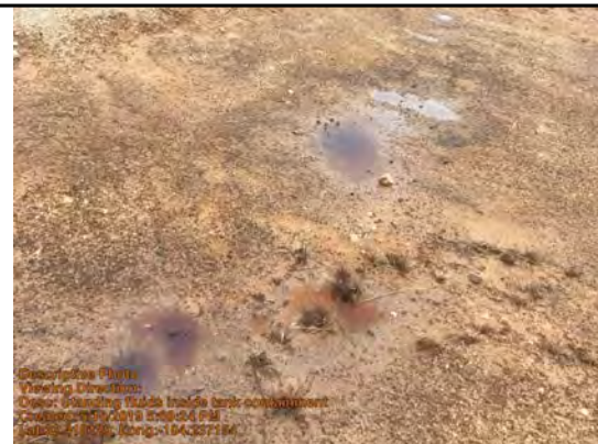
Standing fluids inside tank containment
