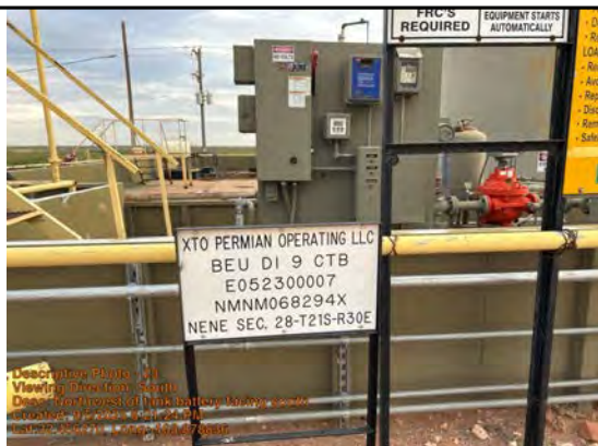
Northwest of tank battery facing south.
