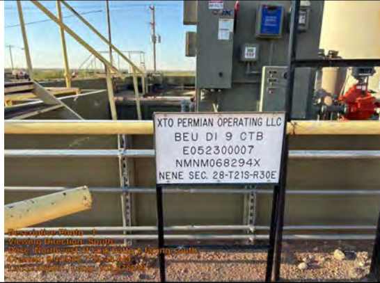
Northwest of tank battery facing south.
