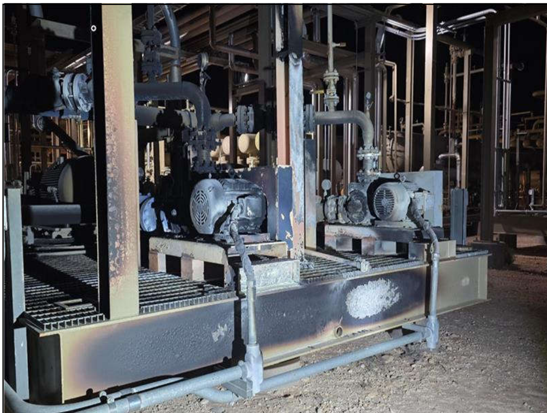
Photo of LPG Booster Pumps facing north.
