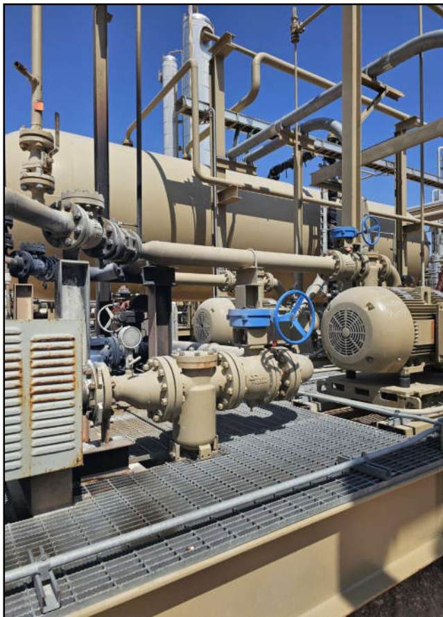
Photo of LPG Booster Pumps facing west.
