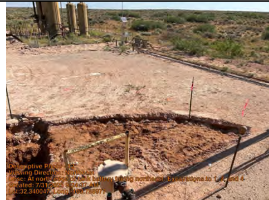
Viewing Direction: Northeast
