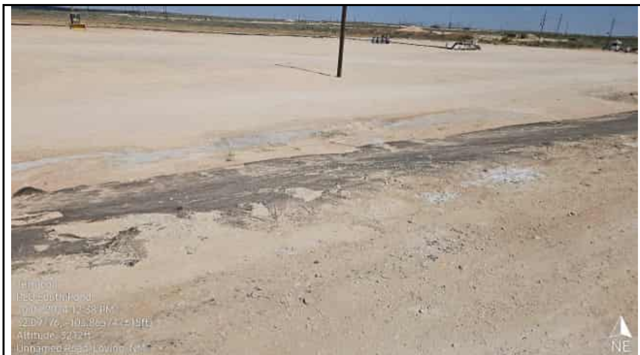
View of the release facing northeast from the top of the pond berm
