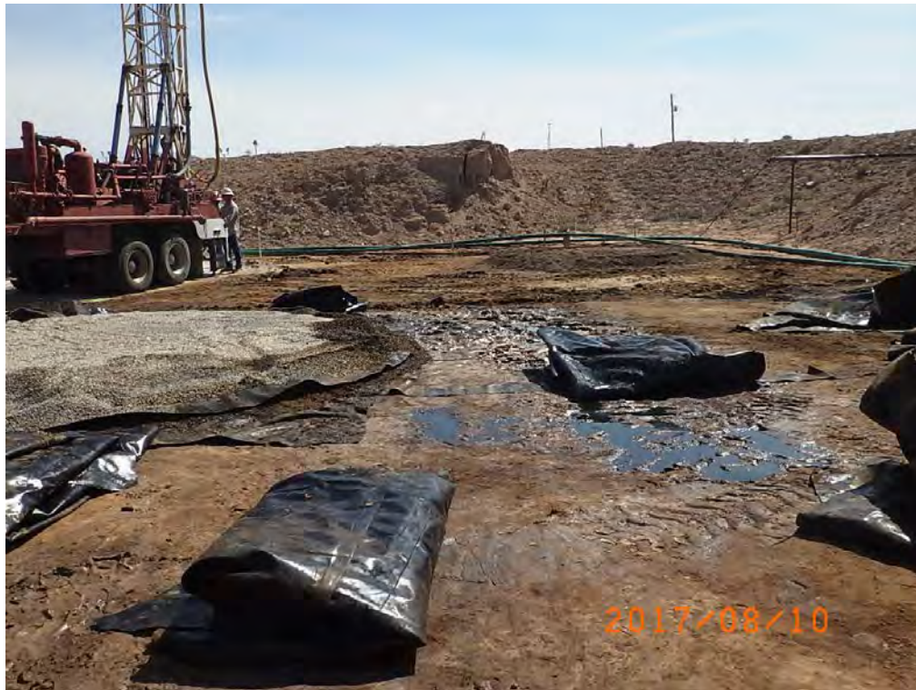
Location Viewing East Prior to Remediation and Chloride Delineation at DP-11, August 10, 2017
