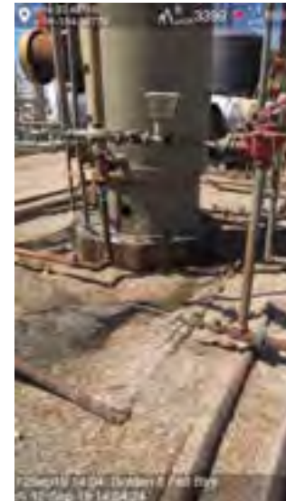
Photograph 8: Surficial staining before hand shoveling activities.
