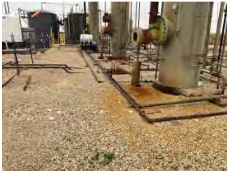
Photograph 3: Surficial staining between equipment.
