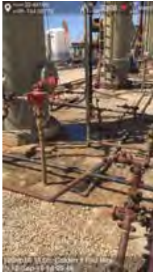
Photograph 1: Northwest view of release staining between equipment.
