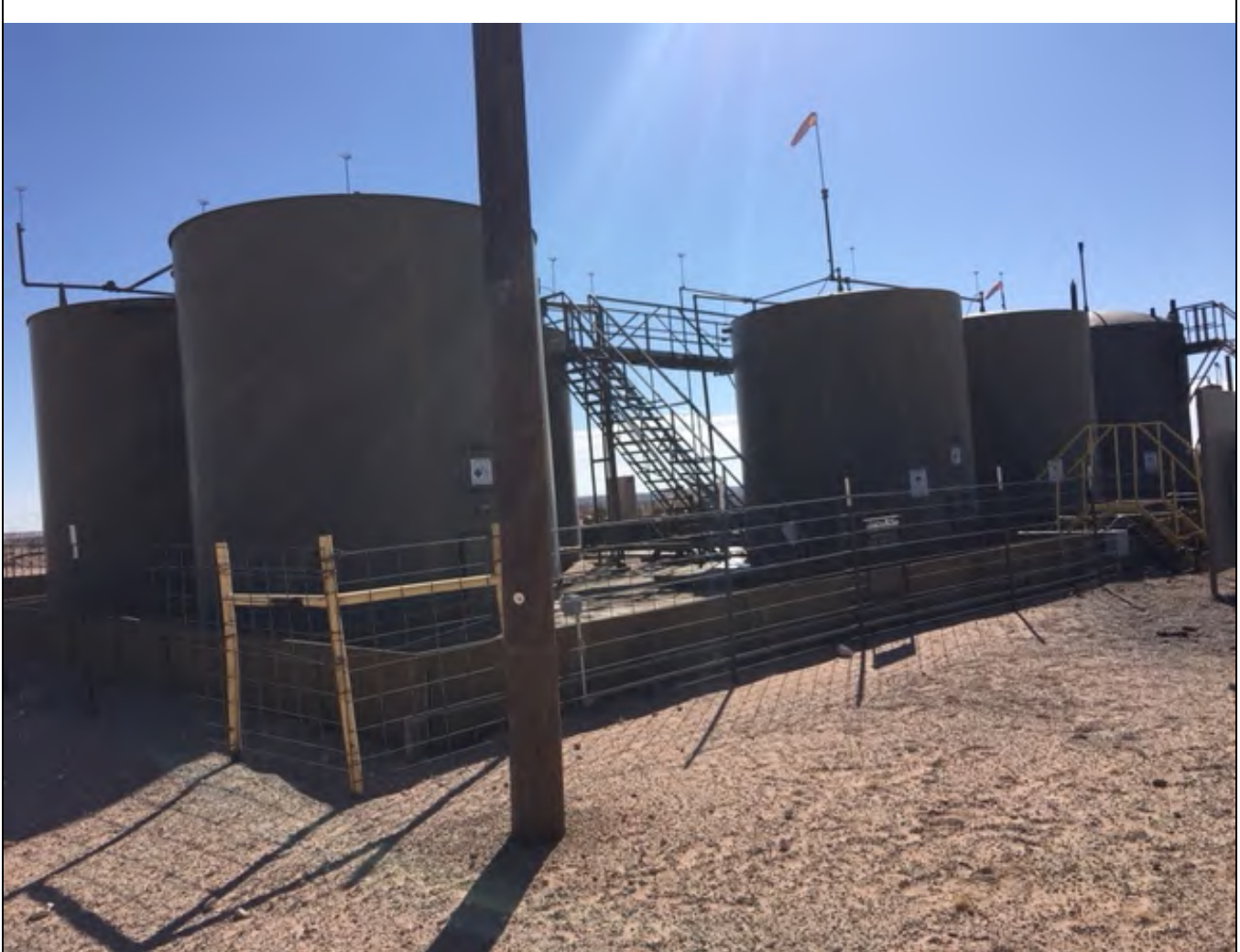
Western view of lined tank battery containment.
