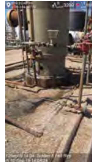
Photograph 8: Surficial staining before hand shoveling activities.
