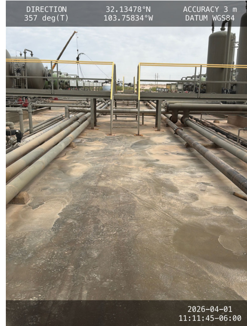
Photo 10 Photo of containment towards north.
