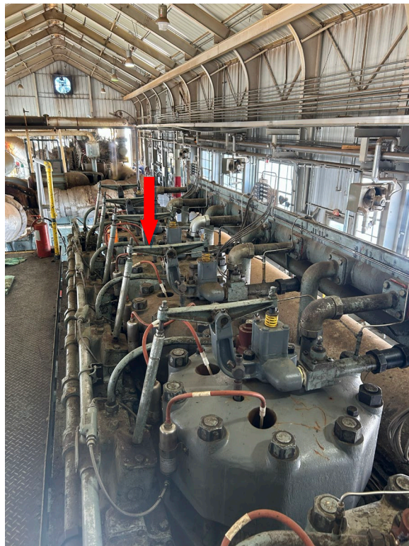
Photo 2: View of where the flash fire occurred.
