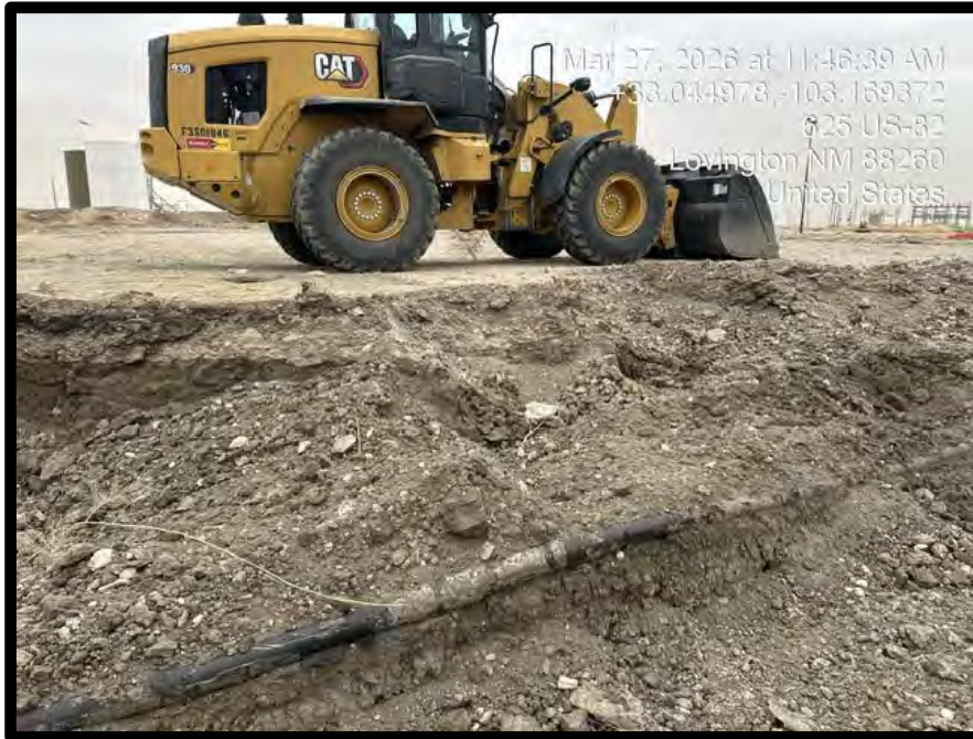
PHOTOGRAPH NO. 7 – A view of the encountered lines in the remediation area.
