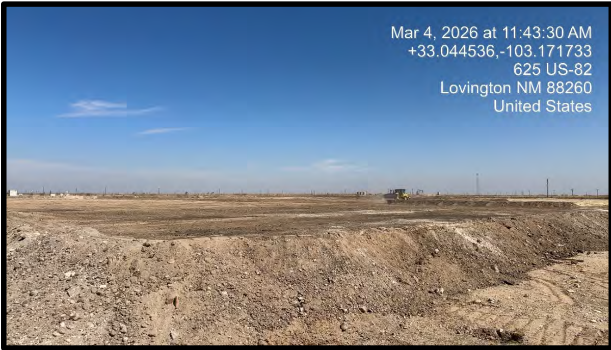
PHOTOGRAPH NO. 1 – A view of the Northern Treatment Cell during the construction process. The view is towards the northeast.
