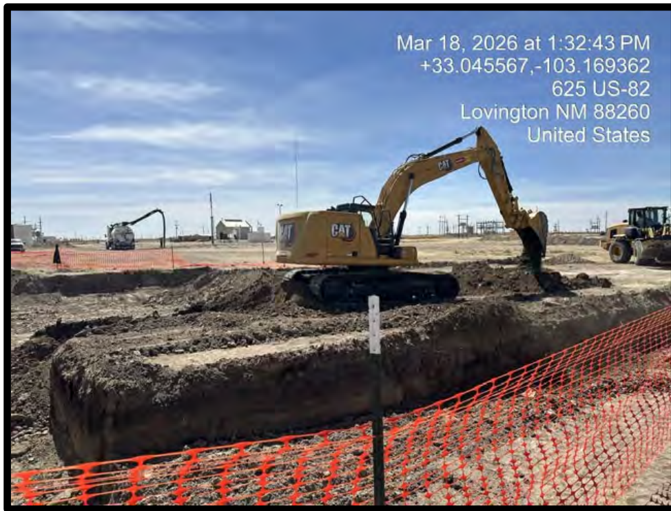
PHOTOGRAPH NO. 2 – A general view of the initial removal operations at the Site. A hydrovac excavator can be seen locating lines in the background of the photograph. The view is towards the south.
