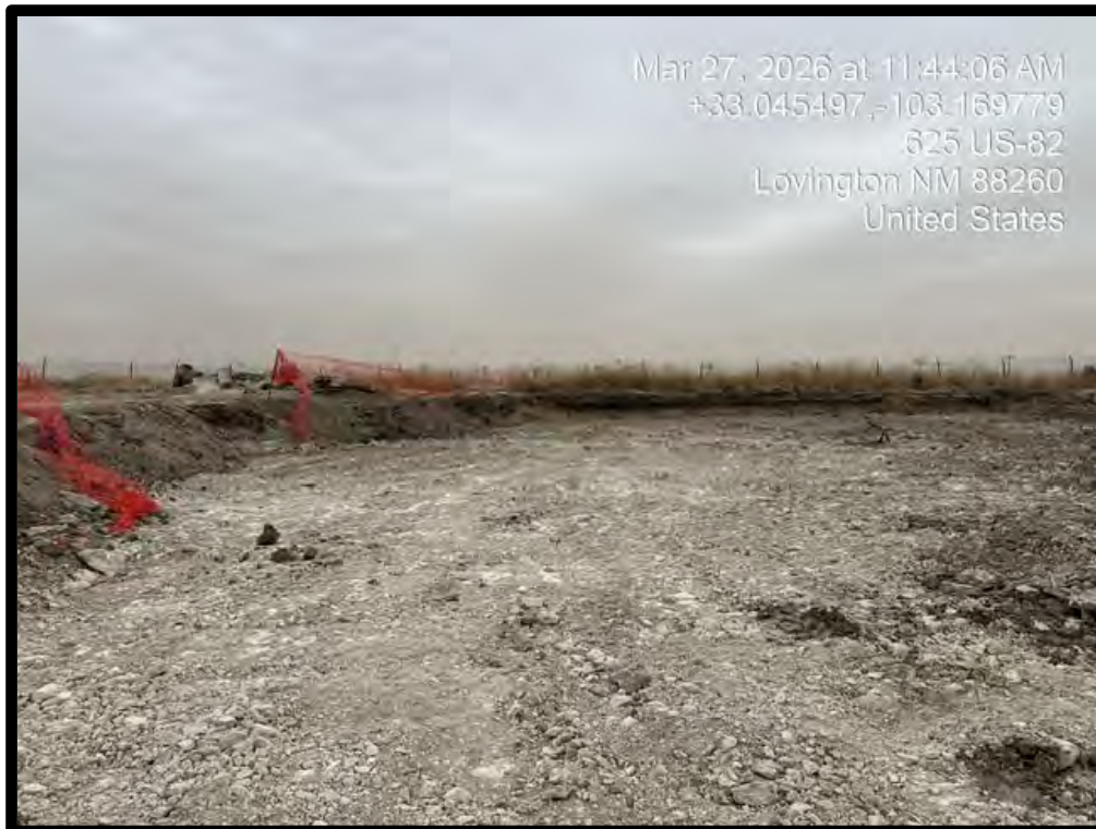
PHOTOGRAPH NO. 4 – A view of the remediation area included in the March 27, 2026 confirmation sampling activities. The view is towards the east.
