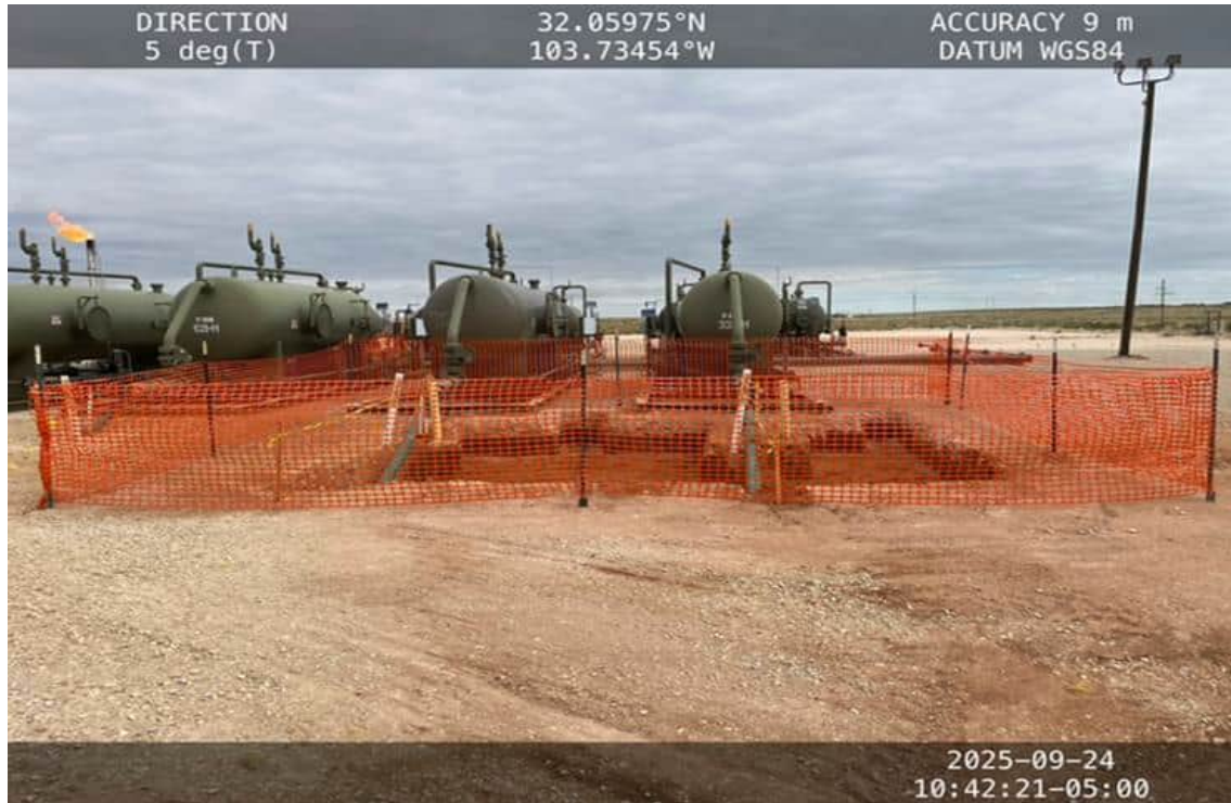
Photo 7 View of excavation adjacent DS-7 sample location facing S from N side.
