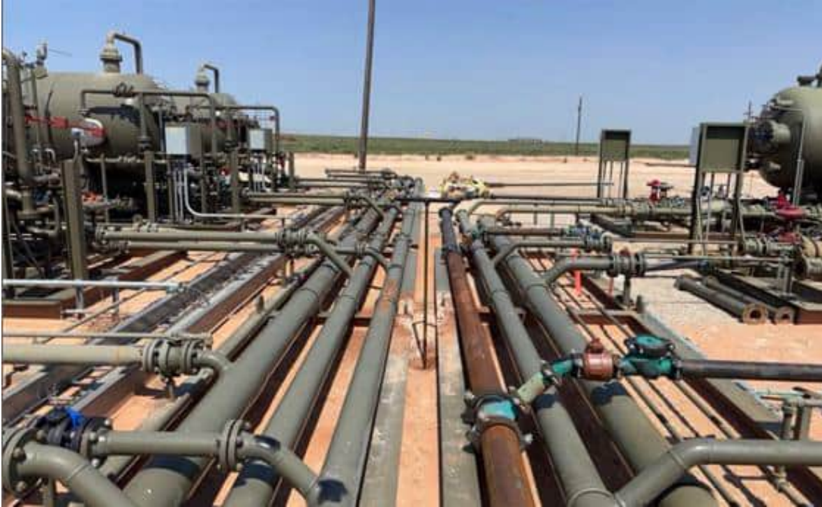
Photo 5 View of DS-1 sample location adjacent to the centralized release area facing E.
