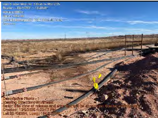
Site view of release and area that will be excavated. Can be visibly seen from staining/orange marking
