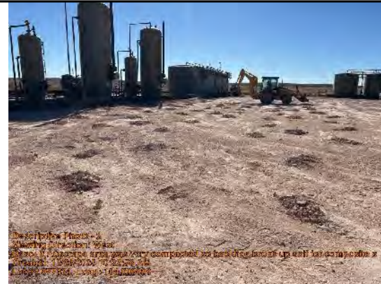
6" scrape area was very compacted so backhoe broke up soil for composite sampling
