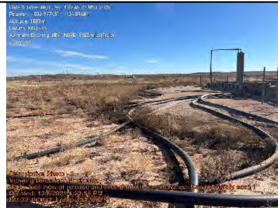
Site view of release and area that will be excavated. Can be visibly seen from staining/orange marking
