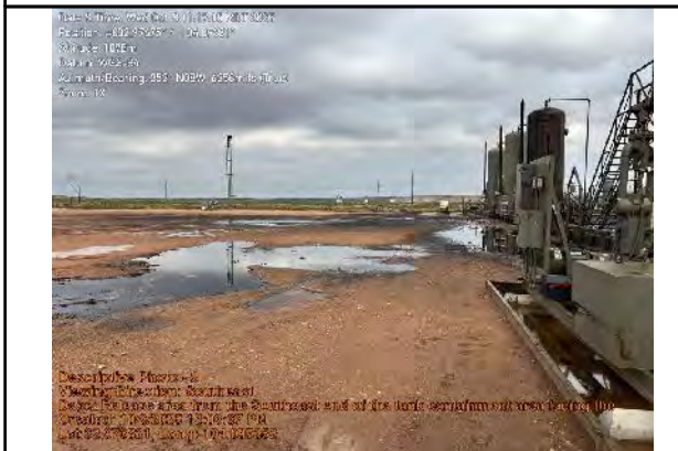
Release area from the Southeast end of the tank containment area facing the pad/heater treater area. Point of source can be seen on the left where heater treaters are covered in crude oil
