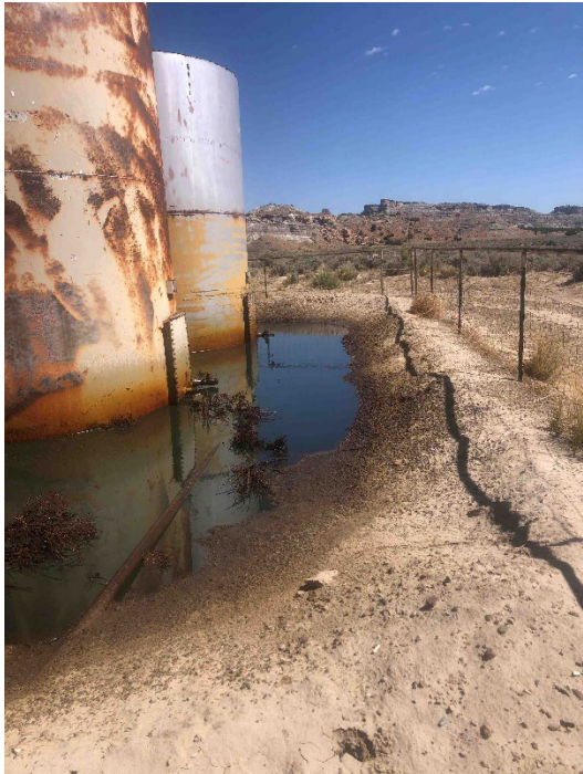
Initial release within secondary containment.
