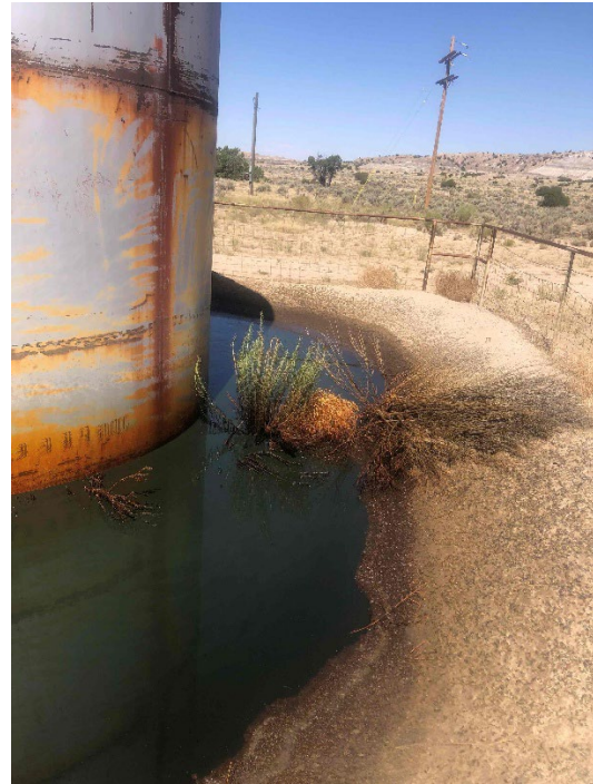
Initial release within secondary containment.
