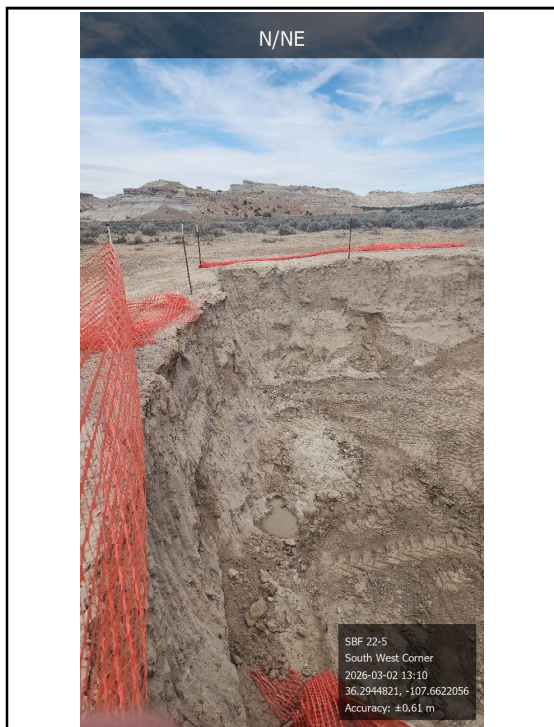
Photo 5 Looking north at the final north wall, west wall, and base of the excavation.
