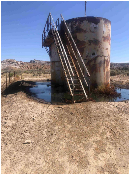
Initial release within secondary containment.
