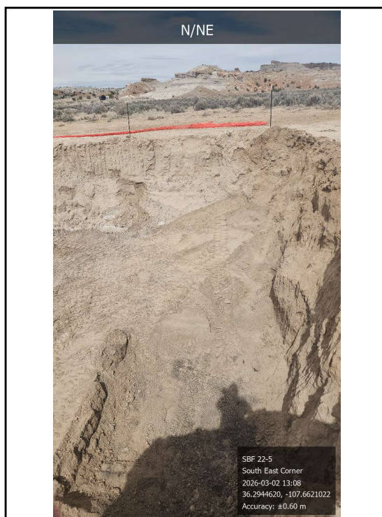
Photo 4 Looking north at the north wall, east wall, and base of the excavation.
