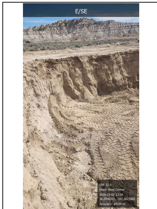
Photo 2 Looking east-southeast at the final east wall and base of the excavation.
