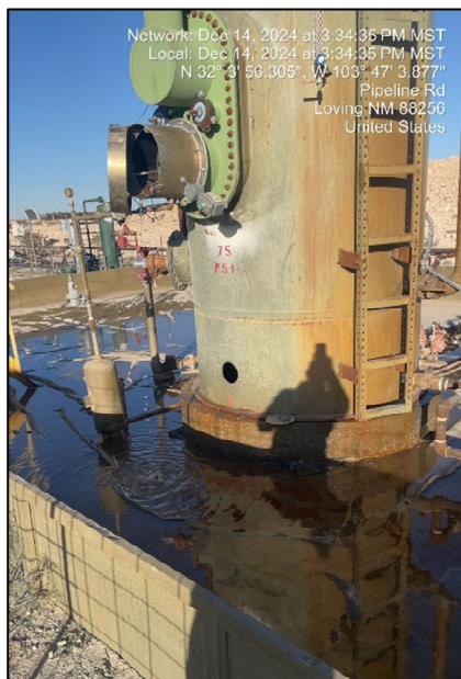
Photograph: 1 Date: 12/14/2024 Description: Initial release extent View: Northwest
