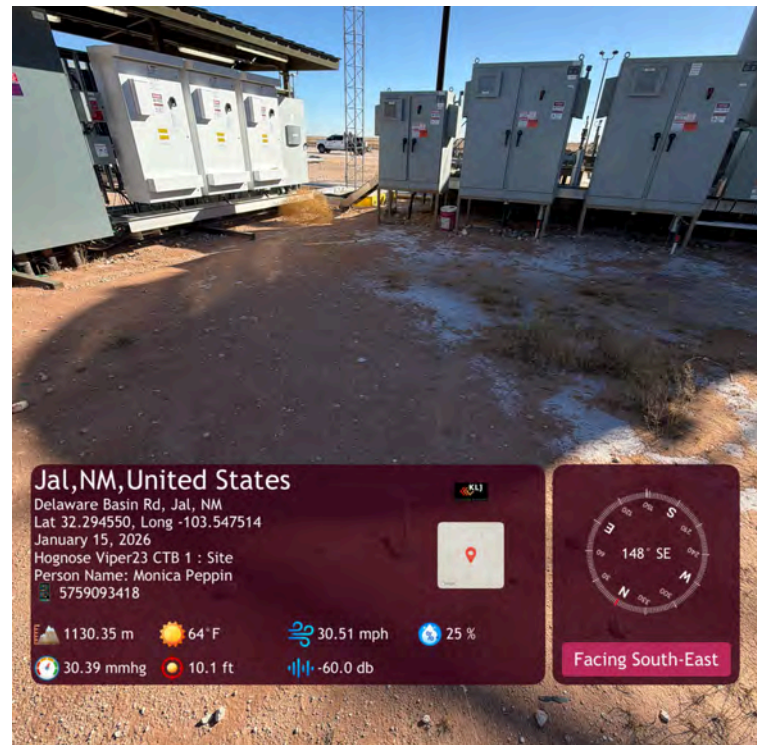
Staining around electrical.
