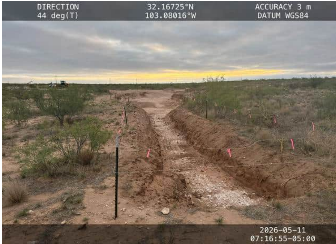
Photo 11 Looking NE at the excavation from the end of the release in the natural drainage
