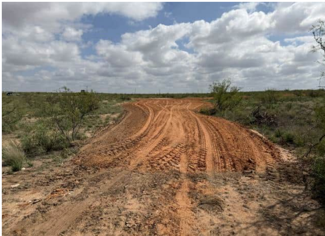
Photo 12 View looking NE from the end of release at the excavation backfilled.
