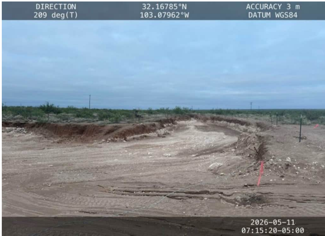
Photo 7 Looking SW at excavation where release entered the natural drainage.
