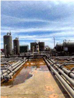
Photo 3 of 5 - Spill Across Pipeline Skid
