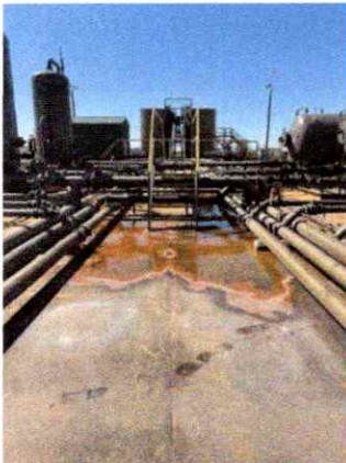
Photo 3 of 5 - Spill on Skid Deck Surface
