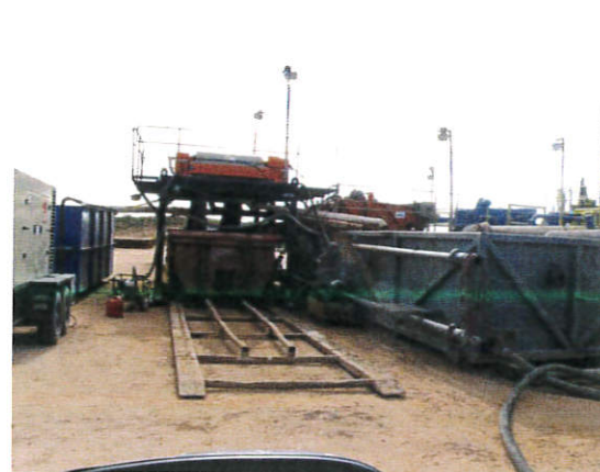
Above: Centrifugal Closed Loop System
