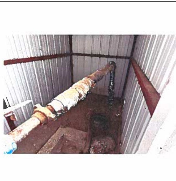
Photograph 4 Date: 5-8-2024 Description: Well head flow line View: NA
