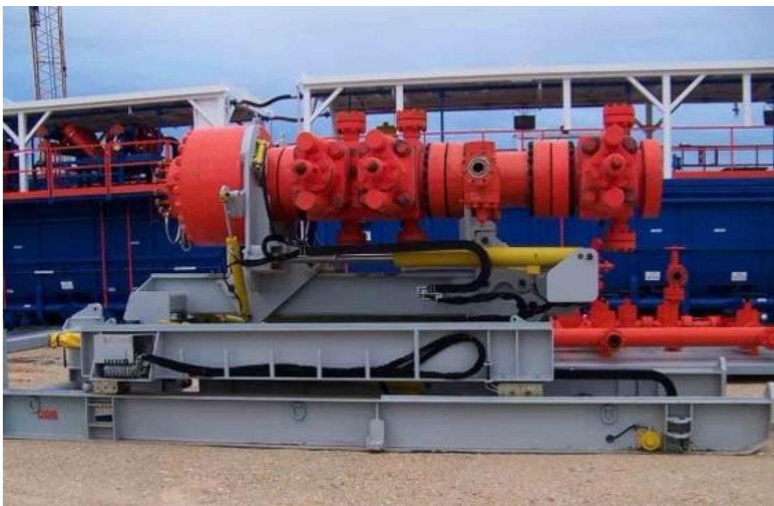
Figure 4. BOP handling system
